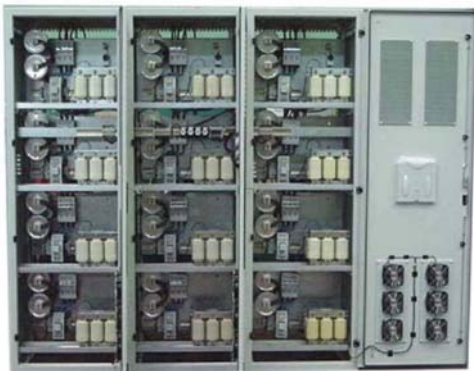
Fig. 2: Detuned PFC system with forced cooling and key components arranged under appropriate thermal conditions.
